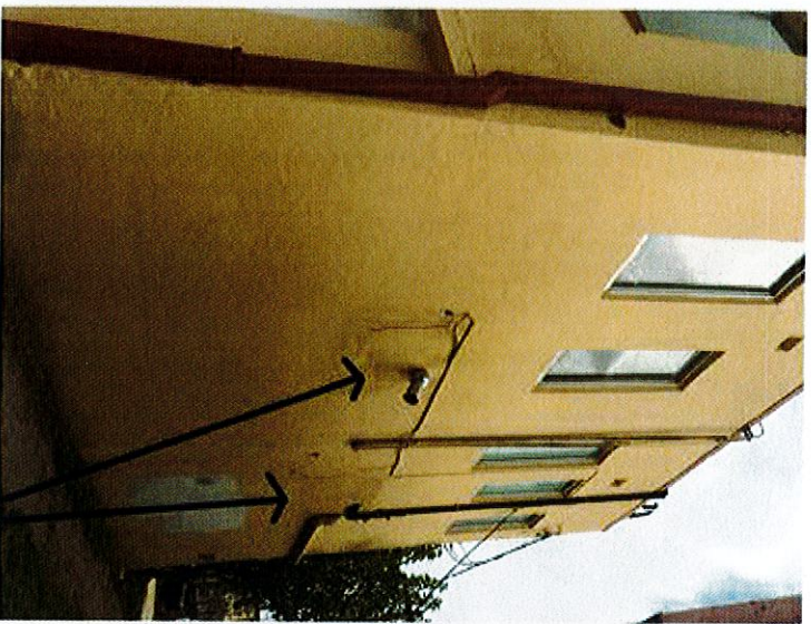
PROPOSED VENT LOCATIONS TO PENETRATE THROUGH ORIGINAL LOWER WINDOWS AT FIRST FLOOR - CURRENTLY INFILLED WITH STUCCO
