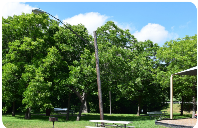
Site lighting near the Santos Arredondo Park. Overall condition is average.
