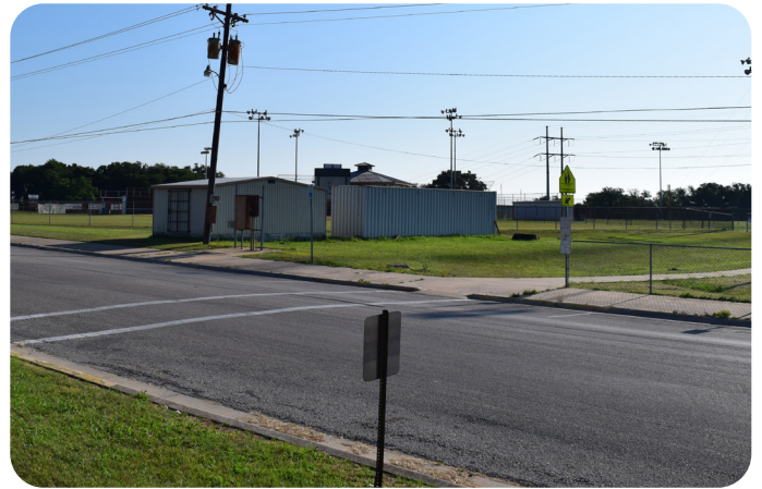
Crosswalk and sidewalks leading into the Youth Sports Complex. Overall condition is slightly average.
