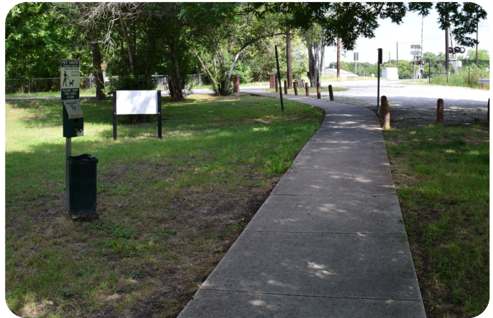
Park pathway from parking lot in Santos Arredondo Park. Overall condition is below average.
